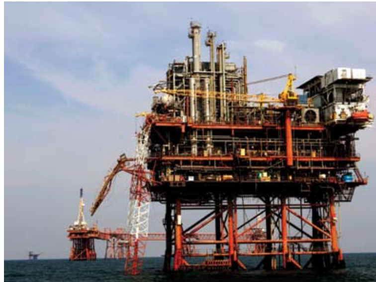
A crane on top of an oil rig lies toppled over on its side after it was damaged by the passage of Hurricane Katrina.
